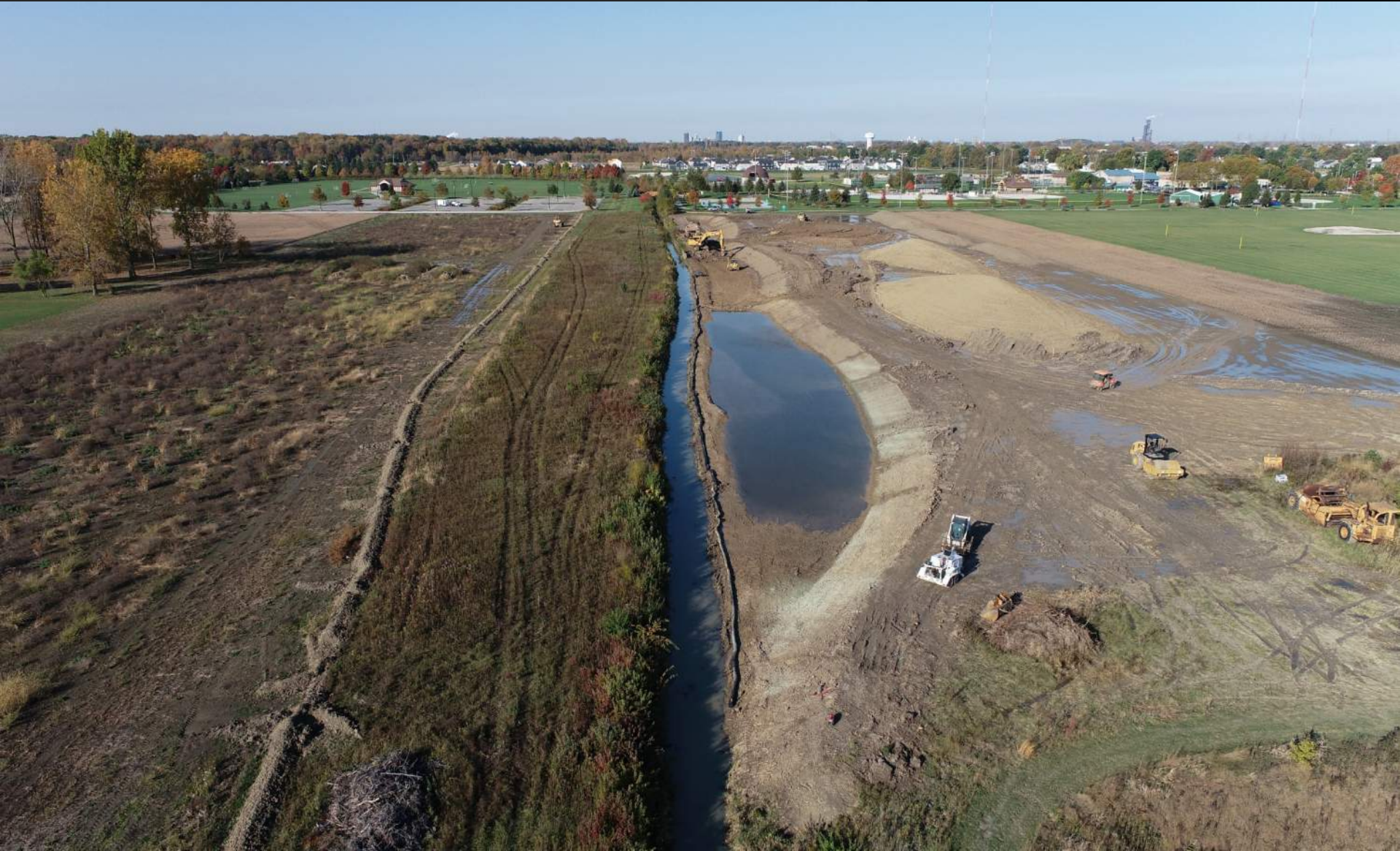
Construction of North Floodplain, Wolf Creek Stream and Floodplain Restoration Project, October 2023
